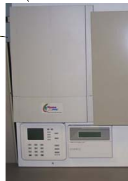
Hidden control and communication components
