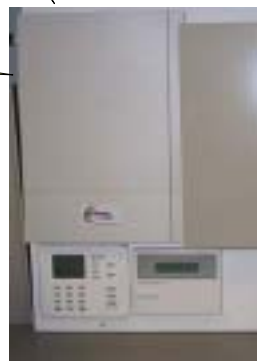
Hidden control and communication components
