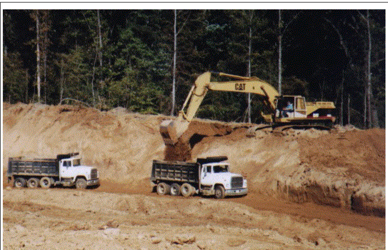
Figure 1: Excavator loading a truck in a mass excavation scenario. The excavator sits on top of an elevated bench, removes the material from the bench, and deposits it into the back of the truck.
