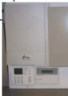
Hidden control and communication components
