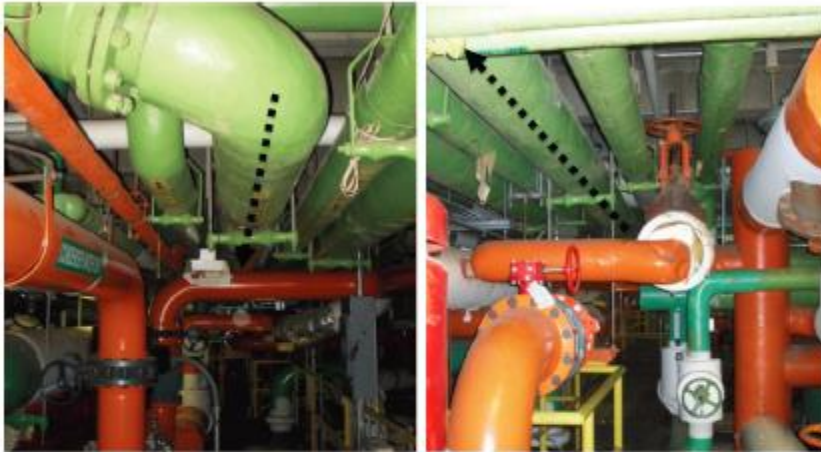
Figure 1. Experiment setup @Wean Hall mechanical space. Pipe with arrow indicates a 10" diameter hot water pipe carrying pressurized hot water flow, on which piezoelectric sensors are installed every 10 ft. A National instruments data acquisition system is used to acquire and store the data for later processing.
