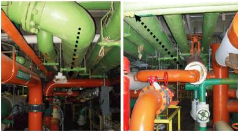
Figure 1. Experiment setup @Wean Hall mechanical space. Pipe with arrow indicates a 10" diameter hot water pipe carrying pressurized hot water flow, on which piezoelectric sensors are installed every 10 ft. A National instruments data acquisition system is used to acquire and store the data for later processing.
